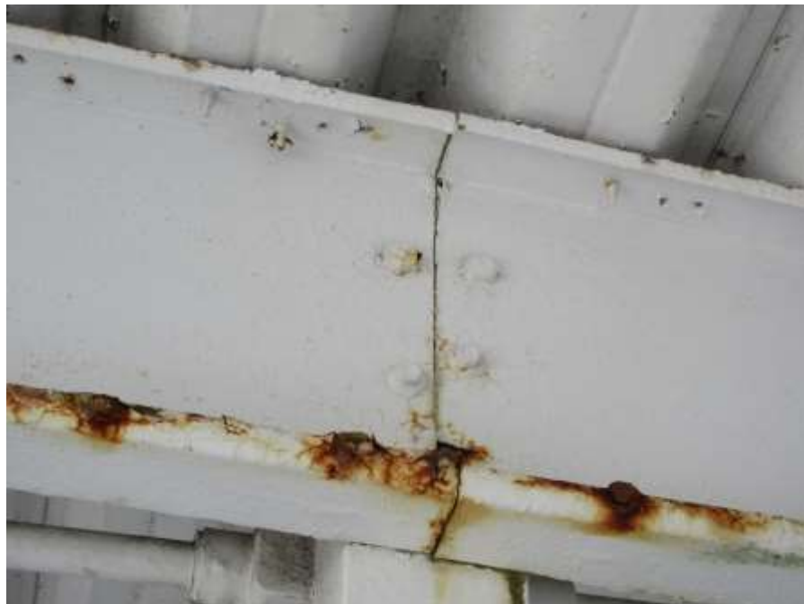
Photo No. 18 – Rusted steel section and connection with improper bolt spacing
