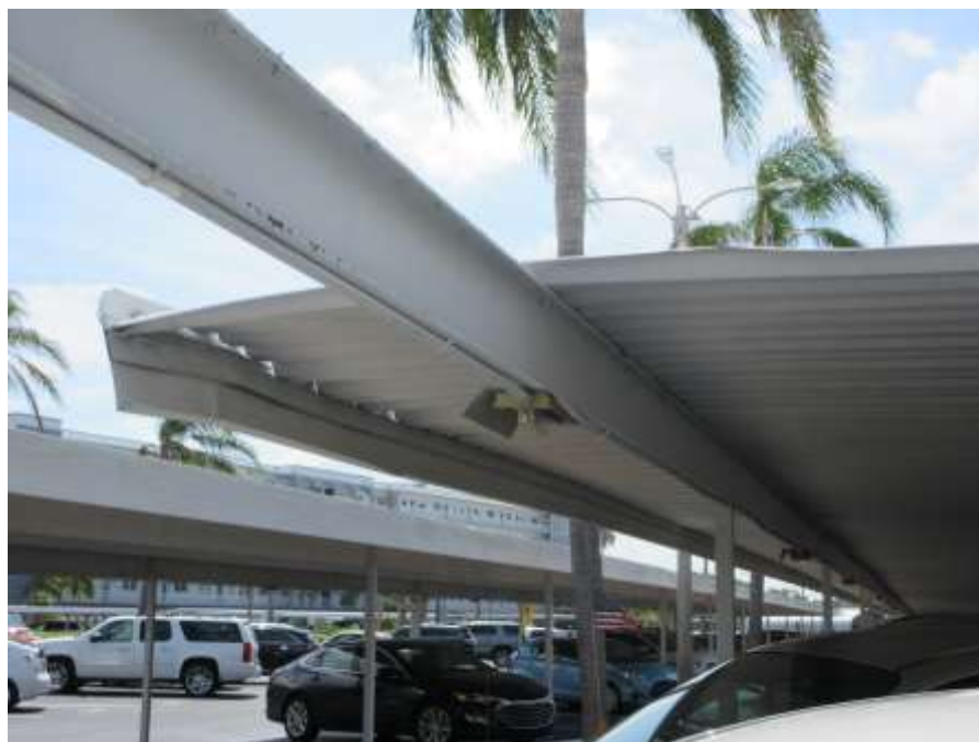
Photo No. 25 – Electrical conduits feeding the outdoor lightning devices.
