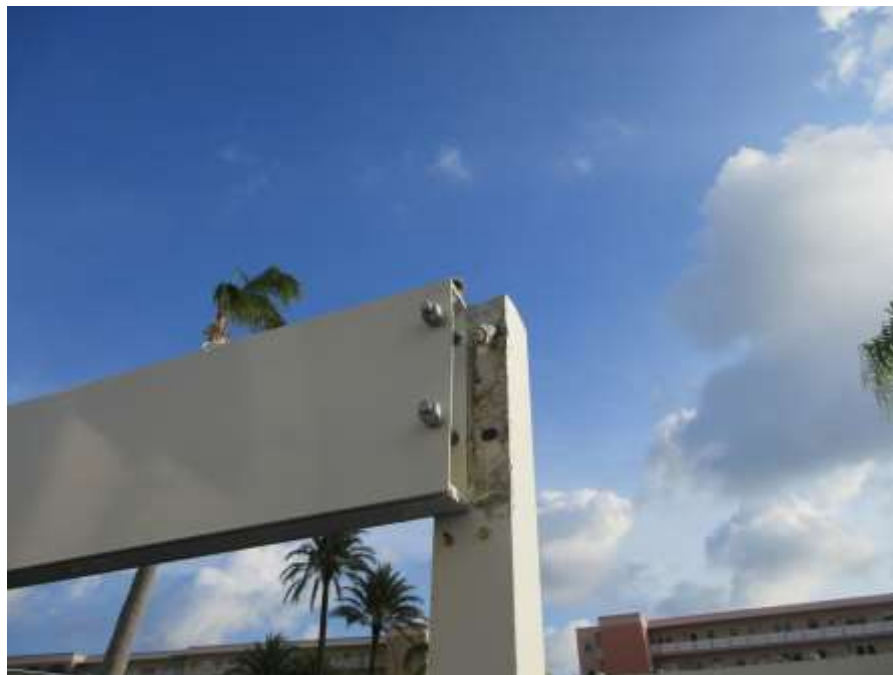
Photo No. 5 – Remaining structure elements showing improper bolt spacing
