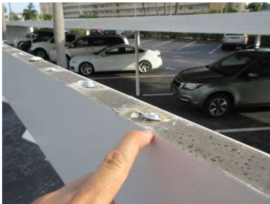
Photo No. 7 – Evidence of panel shear failure
