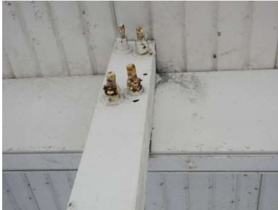
Photo No. 21 – Rusted bolts and inappropriate bolt spacing at connections
