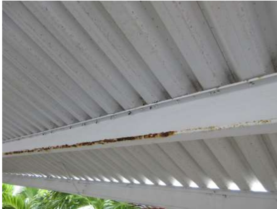
Photo No. 17 – Rusted beam supporting the roof framing of the carport.
