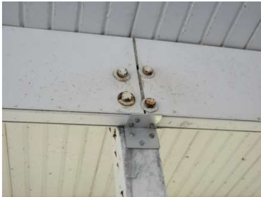
Photo No. 22 – Rusted bolts and inappropriate bolt spacing.
