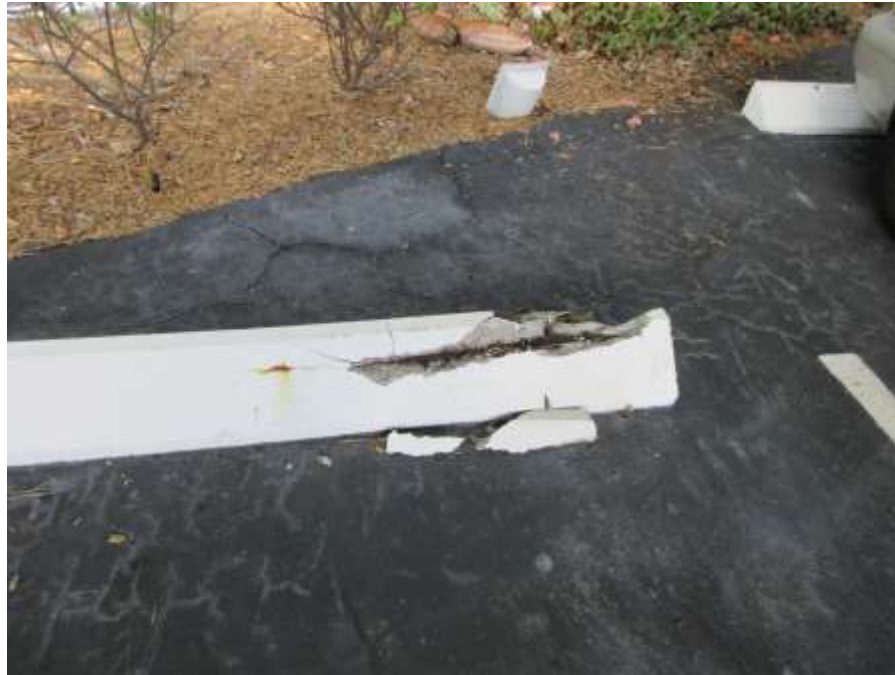
Photo No. 19 – Damaged parking lot blocks (TYP.)
