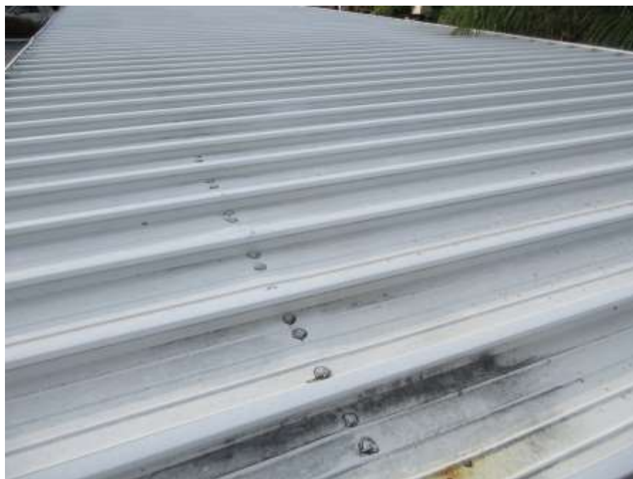
Photo No. 2 – Top view of carport. Evidence of stains from water ponding and bad sealant around fasteners.
