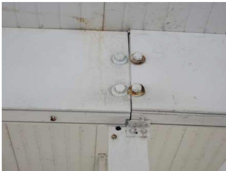
Photo No. 15 – Connection with improper bolt spacing and rust (TYP.)
