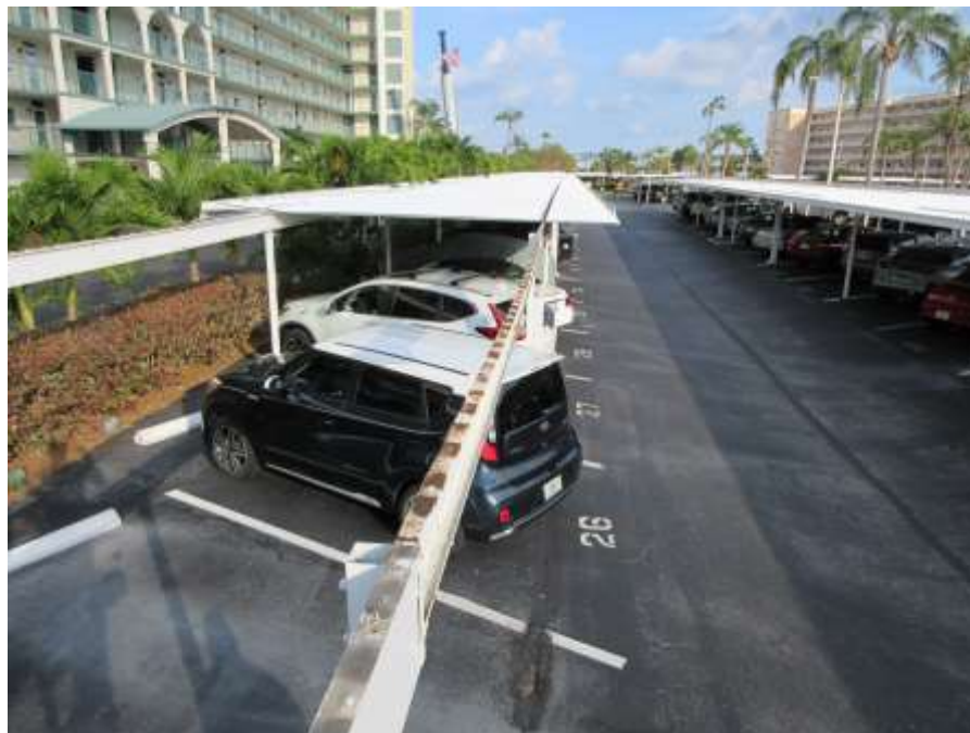
Photo No. 1– Missing/damaged section of the carport from previous hurricane season.
