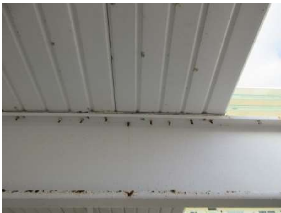
Photo No. 4 – Metal sheet improperly attached to Corroded beam with rusted fasteners.
