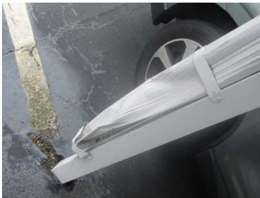
Photo No. 28 – Damaged downspouts showing obstructions in the roof drainage system. New gutters should be placed in areas safe from car collisions.
