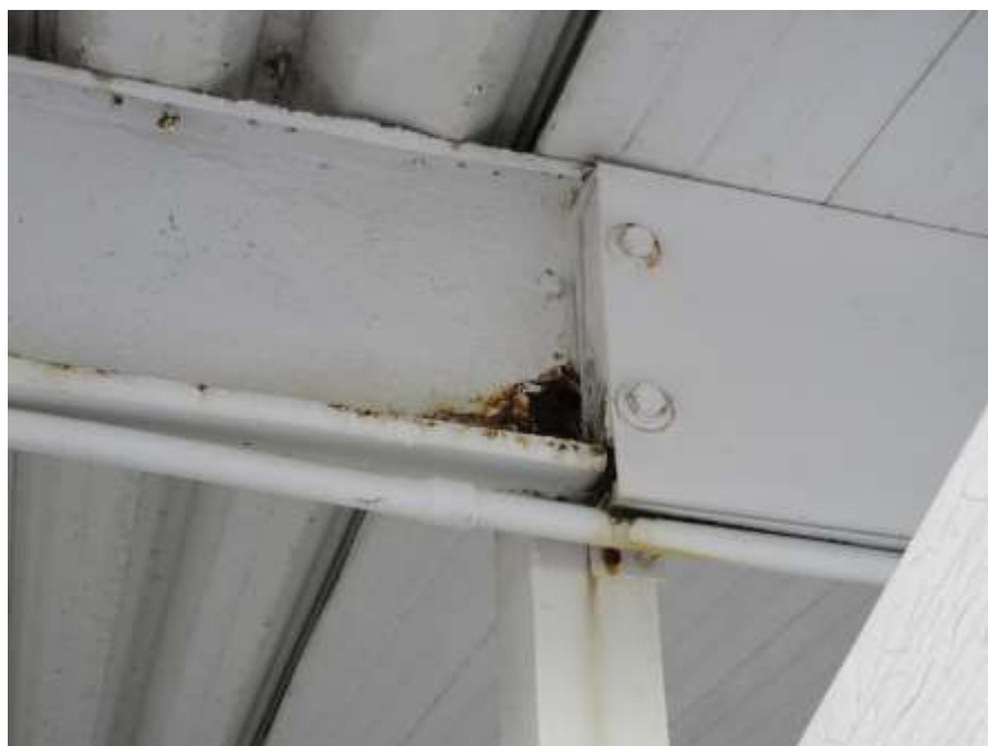
Photo No. 16 – Improper steel-to-aluminum members load connections. I-Beam has loss of section due to rust.
