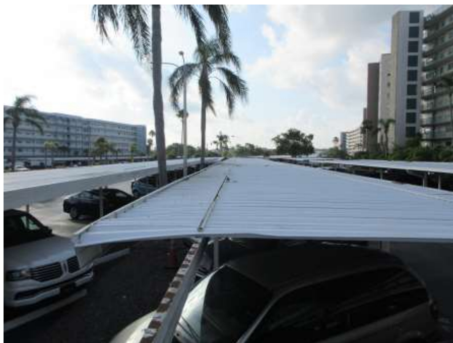
Photo No. 8 – Damages from previous major rain event
