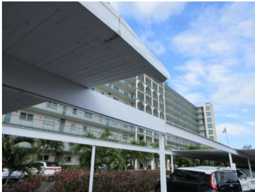
Photo No. 20– Connection of square aluminum section of beam to steel I-beam.
