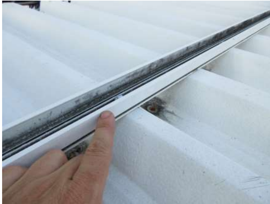
Photo No. 11 – Unused metal sheet support causing more unsealed penetrations in carport's roof. (2)
