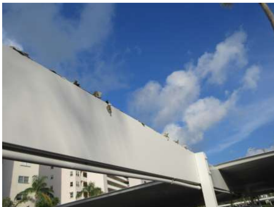
Photo No. 6 – Evidence of panel shear failure
