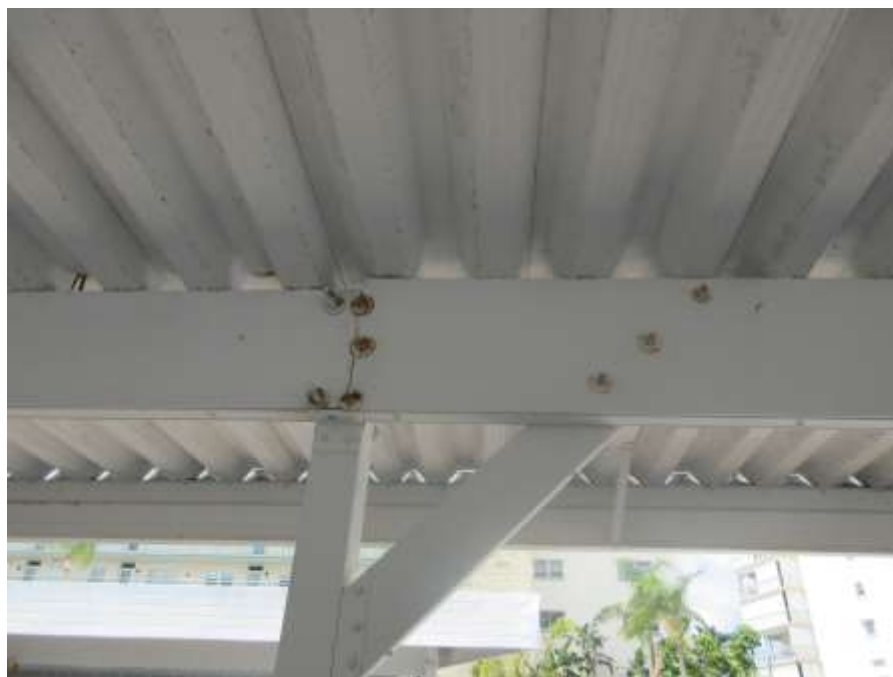
Photo No. 27 – Inappropriate bolt spacing cannot provide the strength required to keep all the components together during a high wind events
