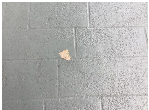
Coating deterioration at the breezeway
