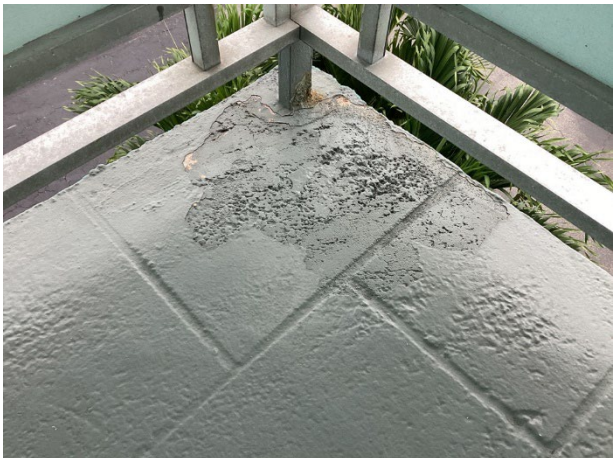
Concrete and coating deterioration at the breezeway
