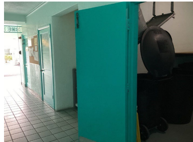
Common area doors
