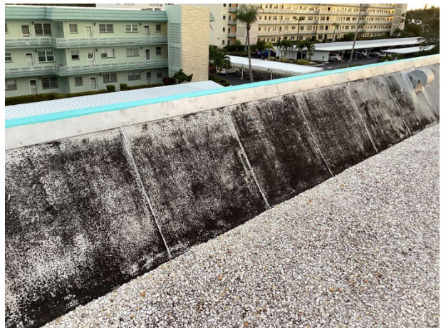
Granular loss at the parapet walls
