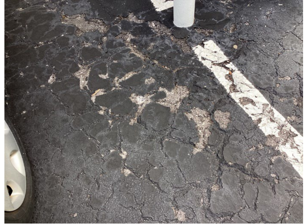
Pavement cracks and deterioration
