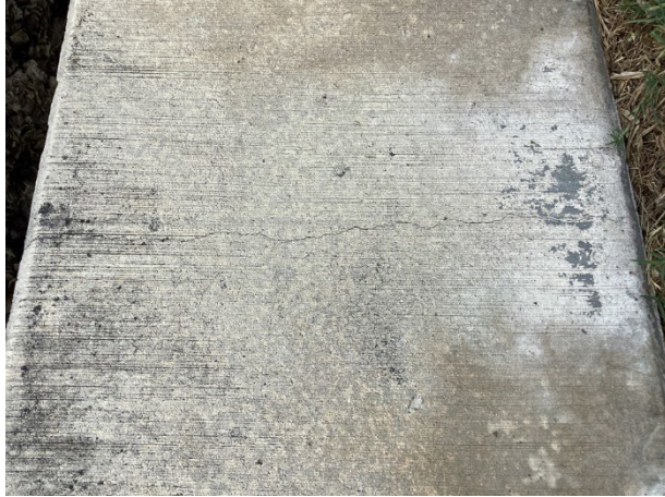
Wall cap with cracks
