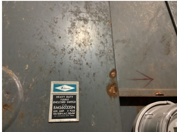
Rust at the electrical panel
