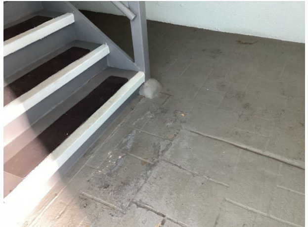
Coating deterioration at the staircase landing
