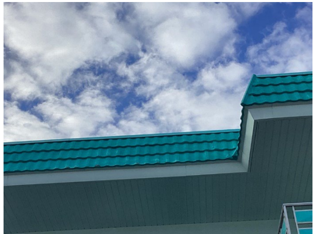
Damage at the metal mansard roof
