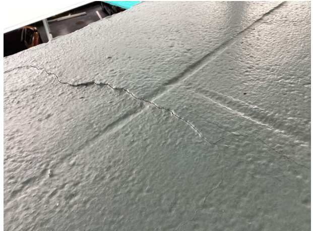
Concrete cracks at the breezeway
