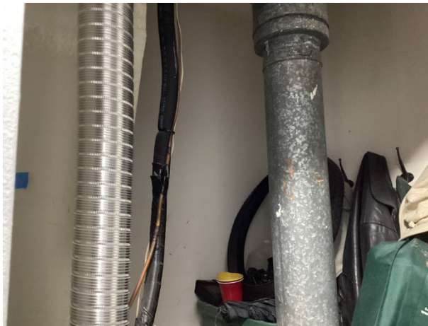
Galvanized steel pipe seen inside the units
