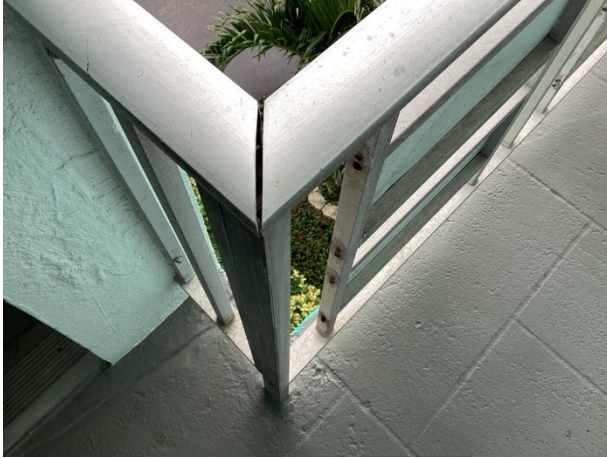
Loose connection at the breezeway railing
