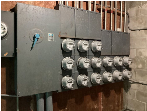
Electrical system components
