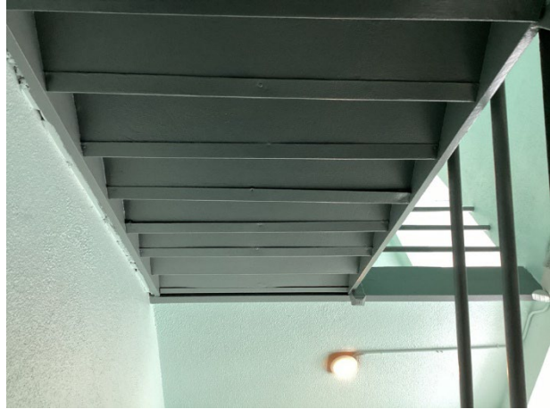
Staircase underside with damage at the wall connection
