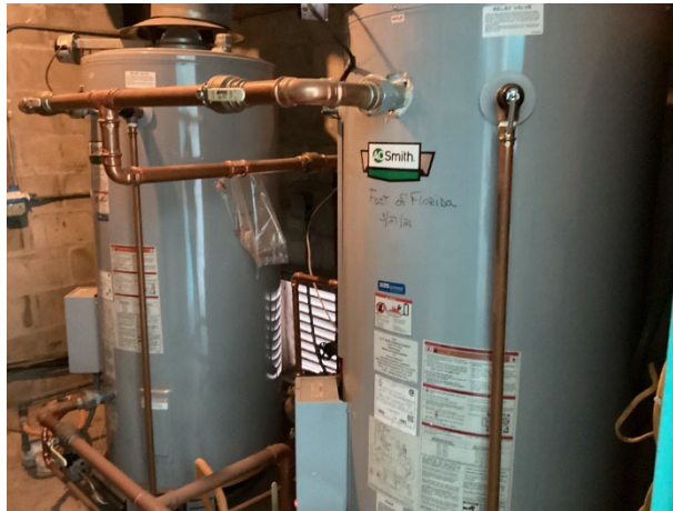
Domestic water boilers
