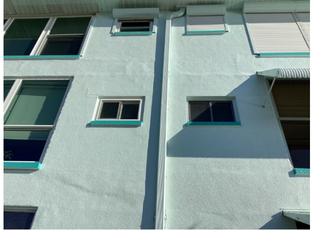
Stucco wall finishes with evidence of minor water intrusion
