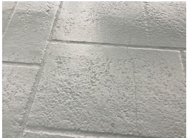
Concrete cracks at the breezeway
