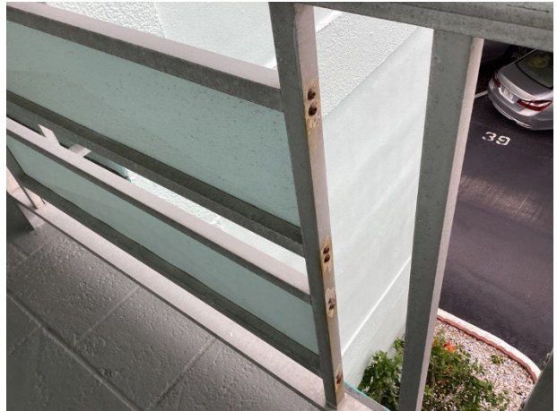
Rusted fasteners and finish fade at the breezeway railings
