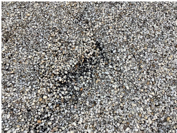
Bare spots in gravel coverage
