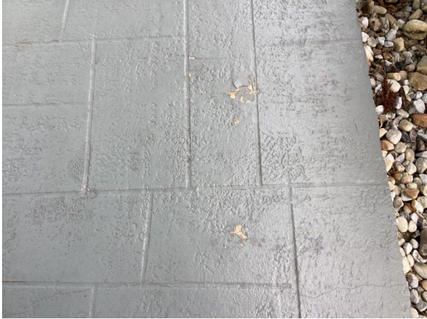
Coating deterioration at the breezeway
