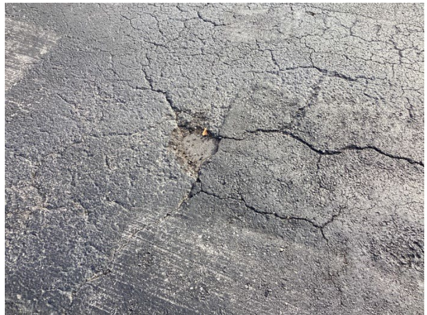
Pavement cracks and pothole formation
