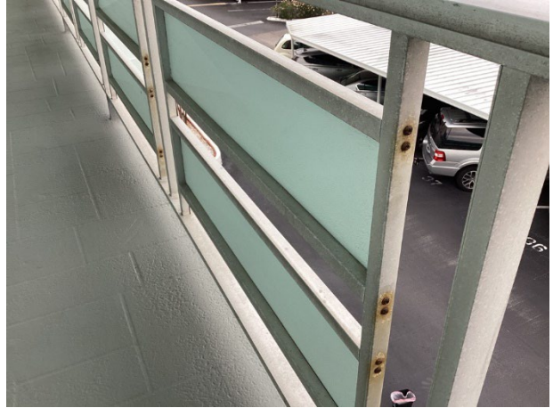
Rusted fasteners at the breezeway railings
