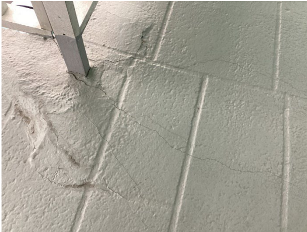
Concrete cracks at breezeway railing attachment
