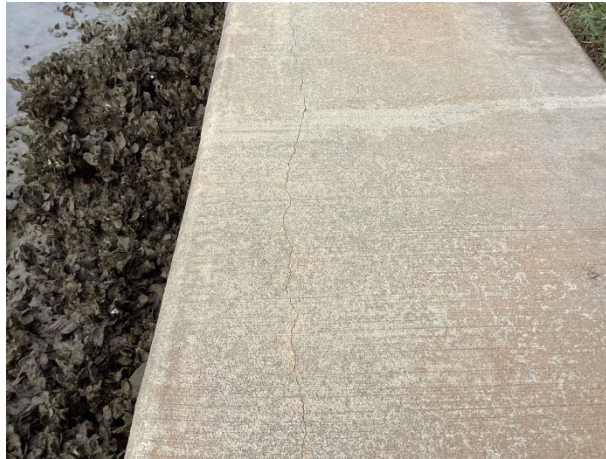
Wall cap with cracks
