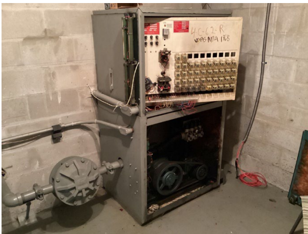
Hydraulic elevator equipment
