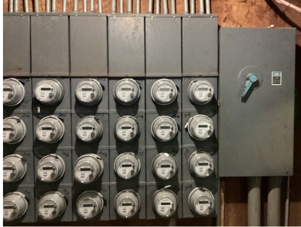
Electrical system components
