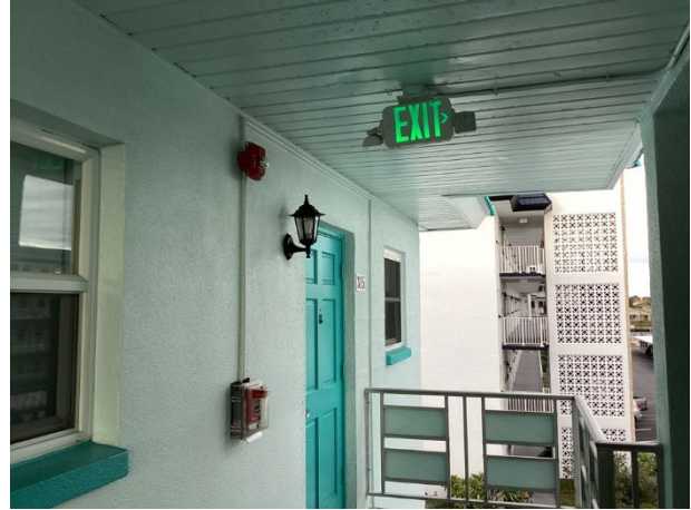
Emergency devices at the breezeways
