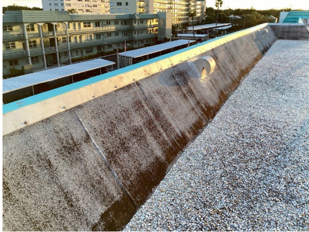
Granular loss at the parapet walls
