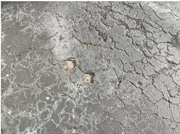
Pavement cracks and pothole formation
