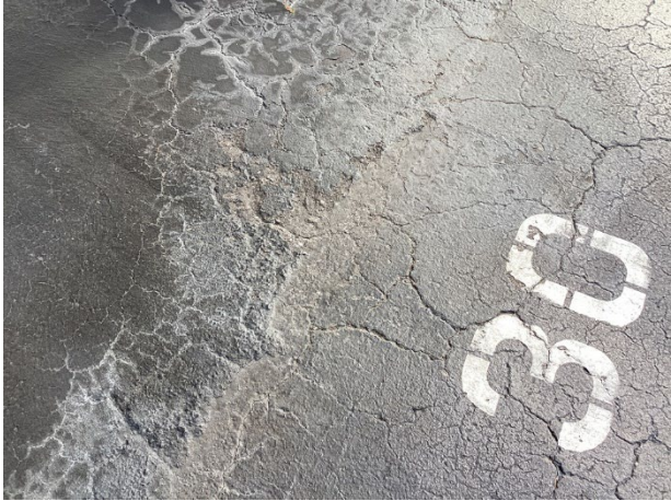
Pavement cracks and raveling
