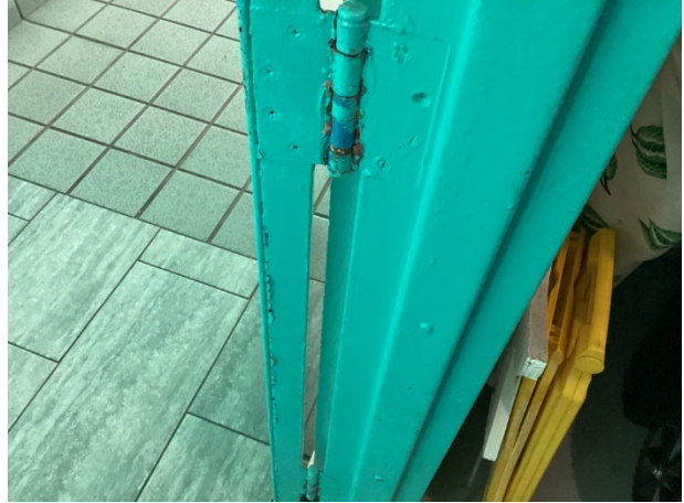
Rust and peeled finishes at the common area door
