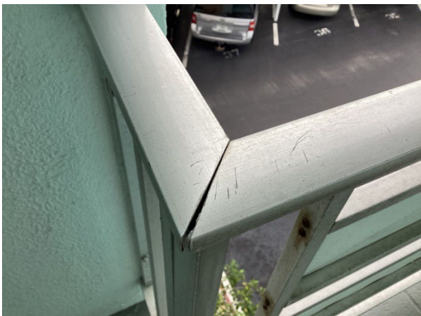
Loose connection at the breezeway railing
