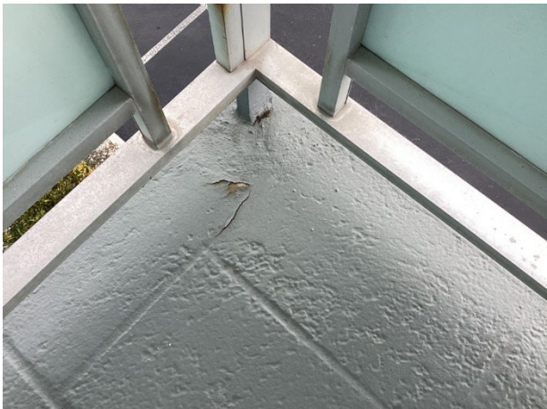
Concrete cracks and coating deterioration at the breezeway
